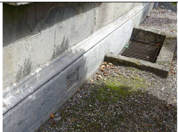
Fig.36: Flaking paint to plinth course to front elevation with flaking paint to air vent.
