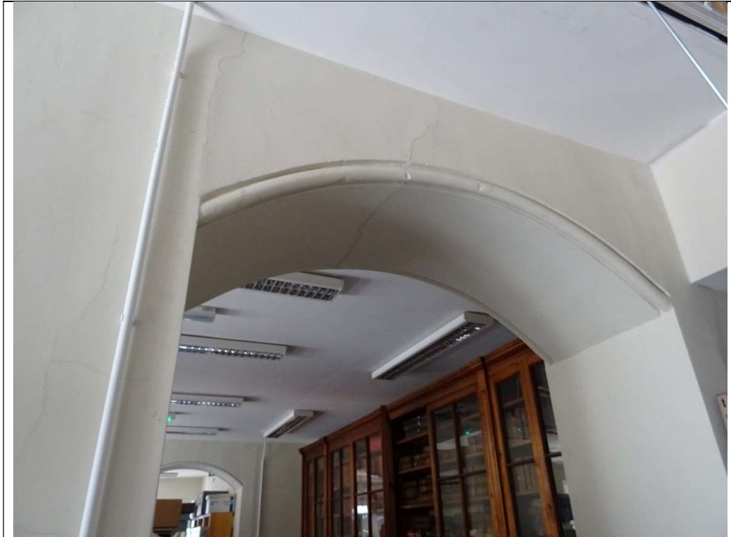
Fig.59: Structural cracking to archway at second floor archive.
