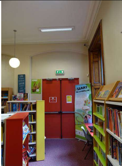
Fig.137: Fire door to east elevation
