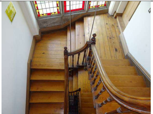
Fig.53: The timberwork of the stairs is by-and-large in good condition. This image shows how the suspension rods support the second half-landing.
