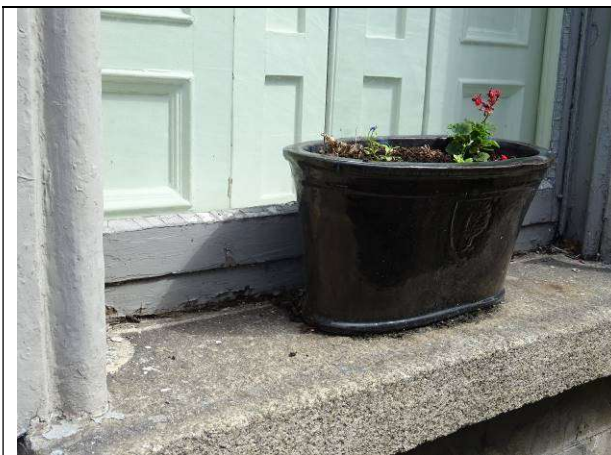
Fig.35: Flaking paintwork to sash with cracked window putty.
