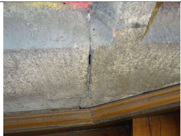
Fig.58: Open joint to ashlar joint of cut-stone granite.
