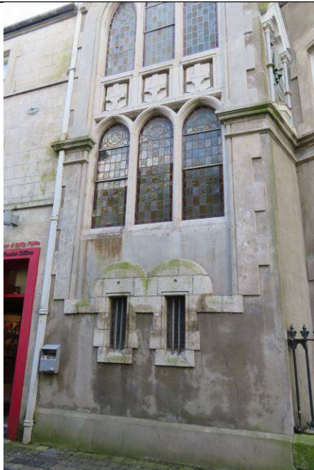
Fig.25: West end with stairs window with saturated render, green and rust staining.
