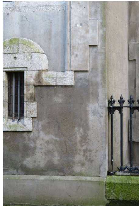
Fig.26: Darker render indicates moisture penetration to render. Any cracks allow moisture to travel inwards resulting in damp penetration.
