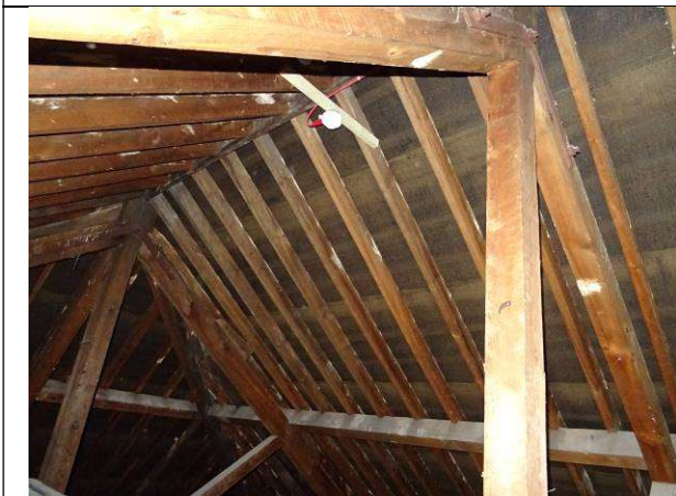
Fig.21: White mould present to timbers below impervious felt.
