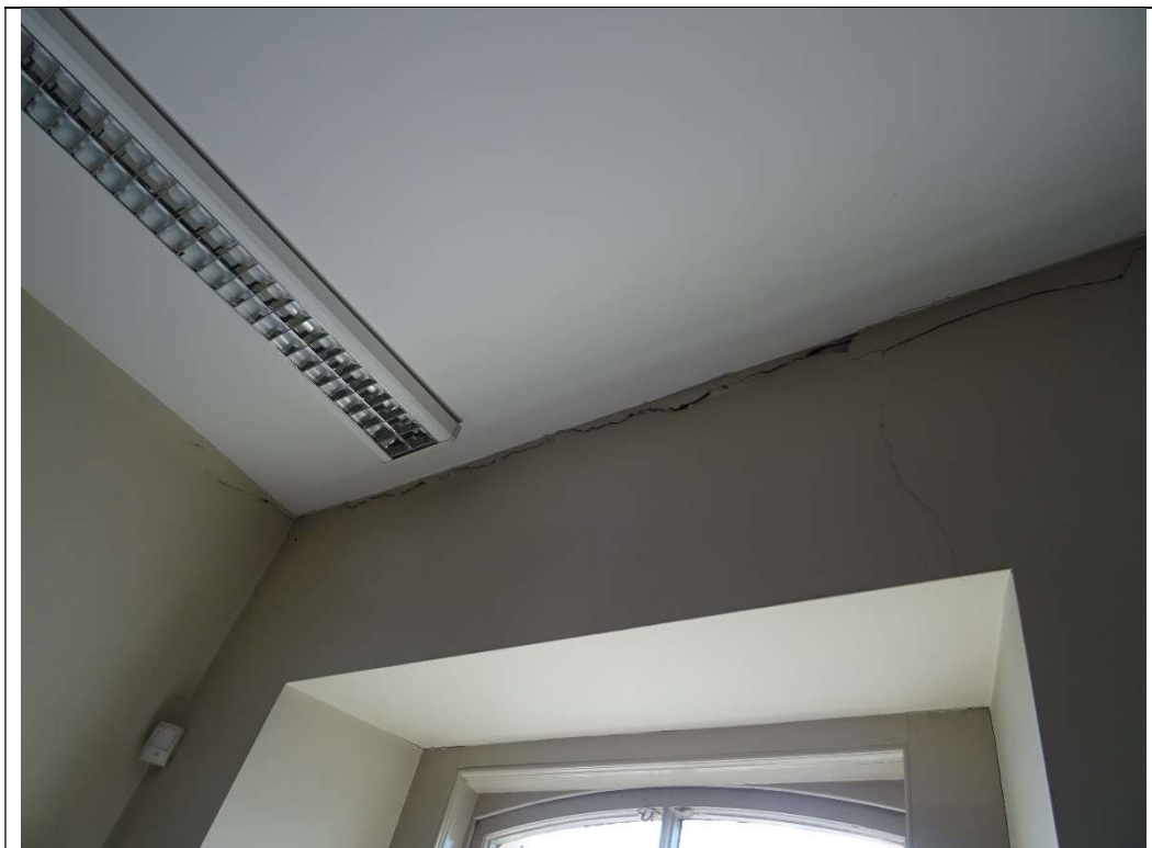
Fig.60: Horizontal cracking to top of front elevation at second floor.
