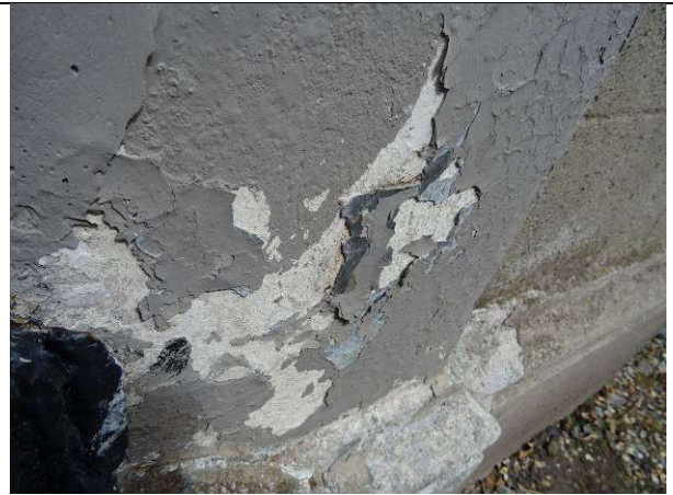
Fig.34: Flaking paintwork to door surround.
