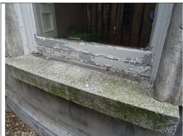
Fig.37: Flaking paintwork to sash window to west elevation.
