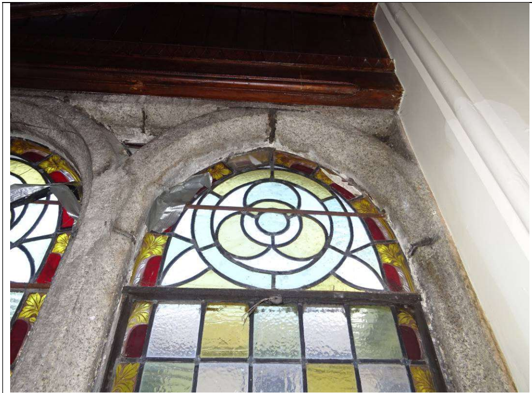
Fig.56: Tape used to secure iron bar. Broken margin panes above.
