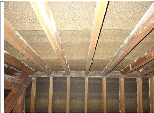
Fig.197: Underside of roof with view up towards ridge board and rafters to either side
