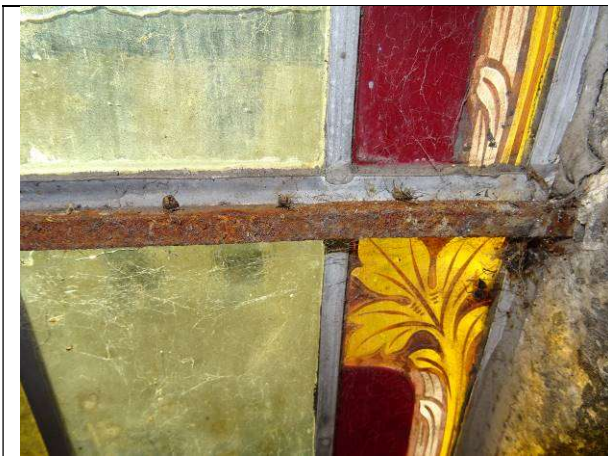
Fig.57: Corroded surface of horizontal iron bar.
