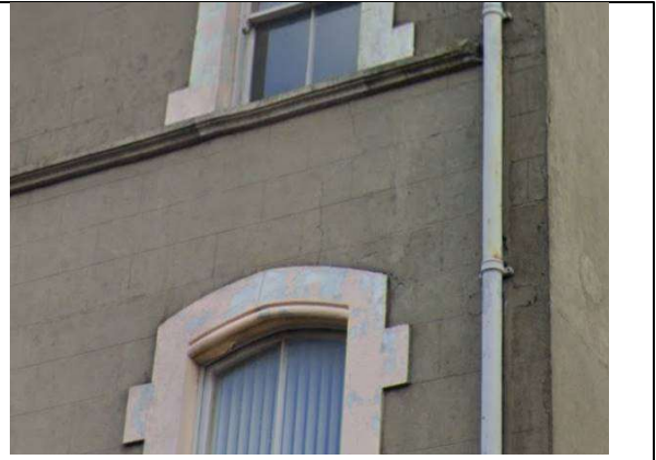
Fig.28: Fine vertical cracks seen in the exterior render of the building. The render has cracked with the slightest of movement because it is so rigid. When rainwater penetrates such cracks, it will not freely evaporate due to the cement render.
