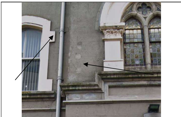
Fig.31: Replacement downpipe with scars of old brackets. Further patch repairs to breakfront render.
