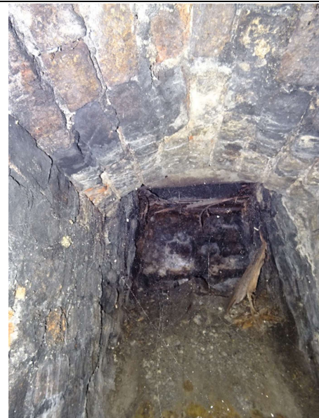
Fig.43: A view up the coal chute towards the inadequately covered opening.
