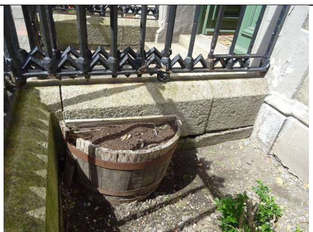
Fig.38: Open joints to stonework and localised corrosion of ironwork to railings.
