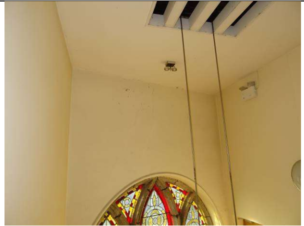
Fig.51: Cracked plasterwork to stairwell. Plasterwork was replaced during renovations.
