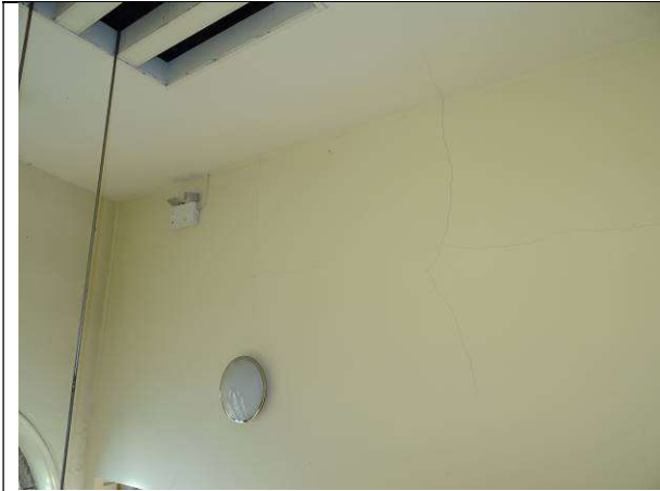
Fig.50: Cracked plasterwork to stairwell. Plasterwork was replaced during renovations.
