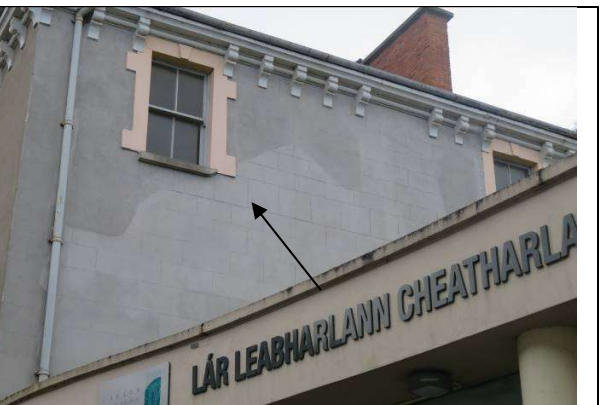
Fig.32: Render applied to the scar of the demolished rear extension. The upper floor windowsill was chamfered to accommodate the roof pitch.
