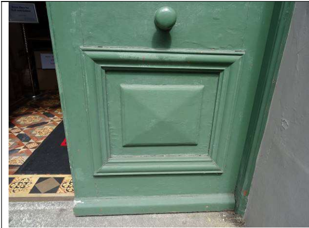
Fig.33: Open joints to bottom panel of door.
