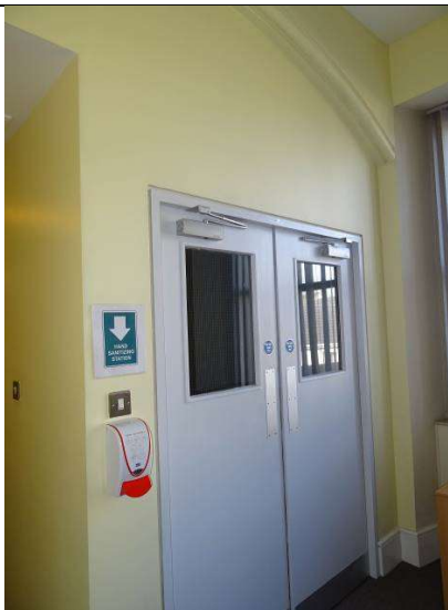
Fig.173: Fire doors to lobby of lift at first floor
