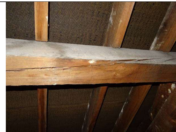
Fig.22: Split along purloin to north side of roof.
