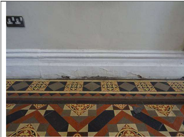
Fig.46: Run-in-situ skirting with flaking paintwork.
