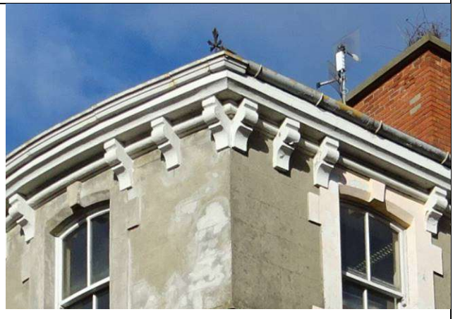
Fig.20: Original flat-bottomed gutter to the bowed west end with a replacement round-bottomed gutter to the façade.
