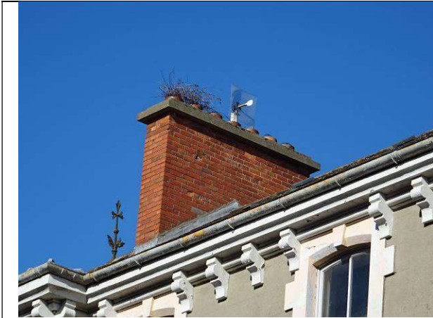
Fig.17: Rebuilt chimneystack with nest material to pots. Spalled brickwork. Cement pointing with cement patch repairs. Flaking paintwork to replacement half-round gutter. Flaking paint to corbels at cornice.
