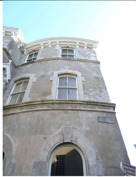
Fig.24: Localised patch repairs to the render at the southwest corner.
