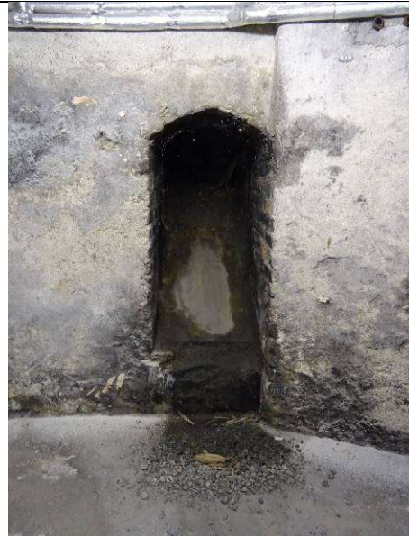
Fig.41: Water is a constant issue for the coal chute located at the west end of the basement. The concealed opening lies beneath the public pavement and allows water to flow freely into the basement.
