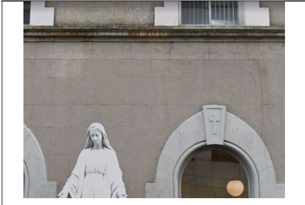
Fig.27: A band of render below the first-floor sill course looks as if it has been renewed. The moulded underside of the sill is very stained by atmospheric pollution. A series of fine cracks can be seen to the render below the upper window.
