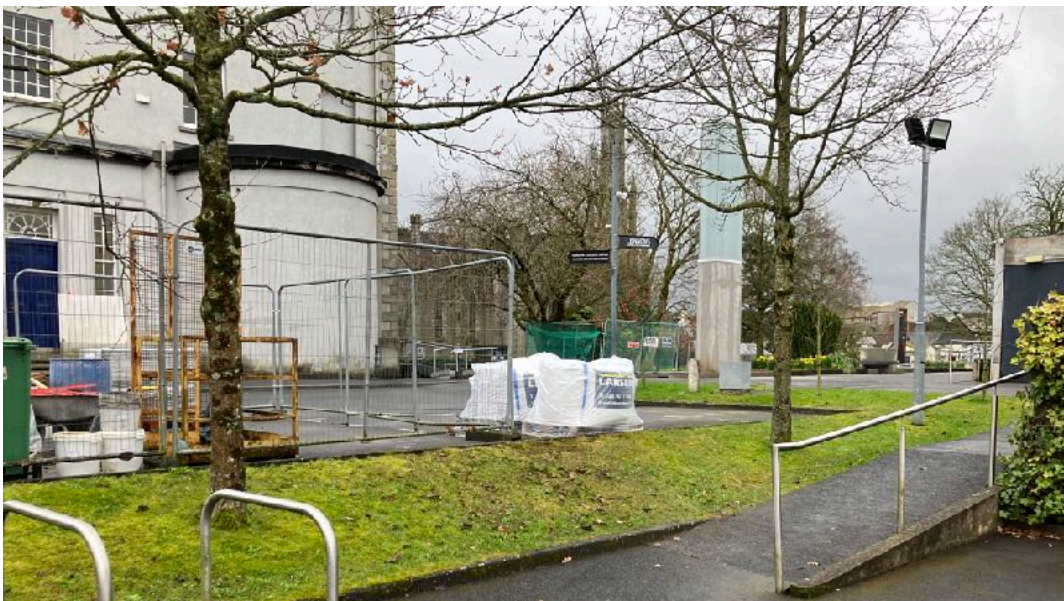
End of new route - west section close to north wing Carlow College
