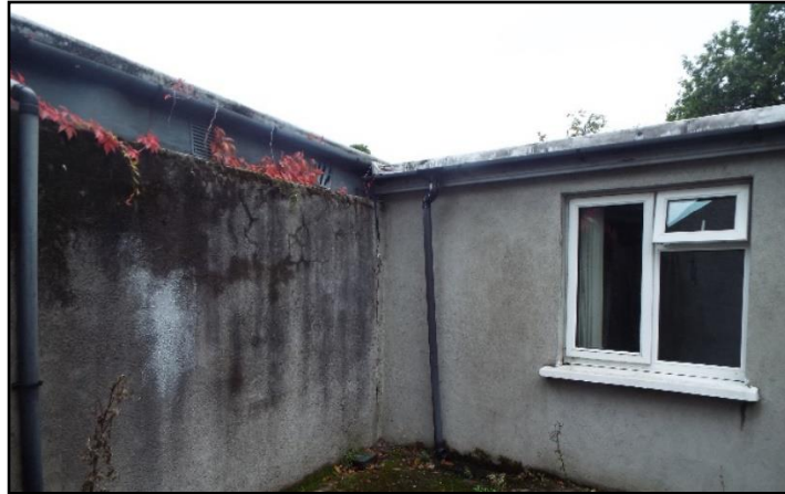
Plate 8: Flat roof areas to be removed (BL3)
