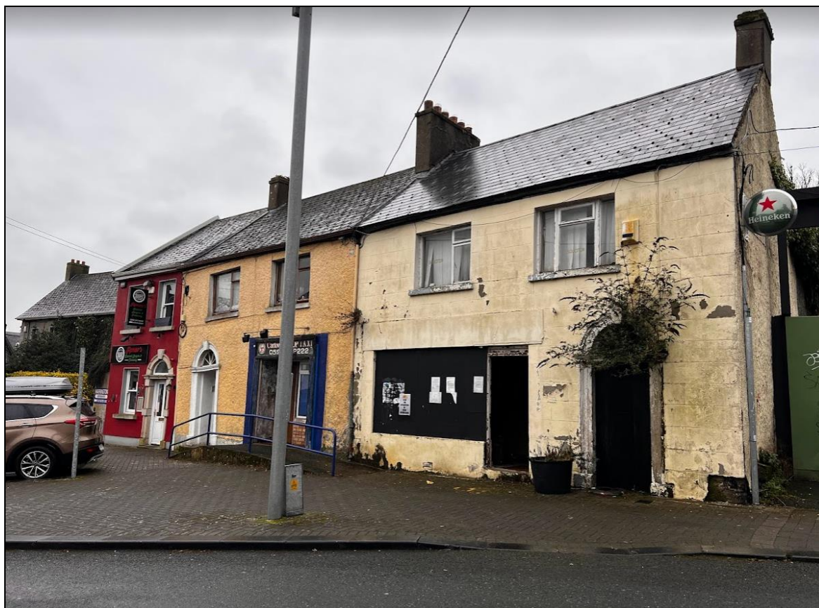
Plate 1: 1 Haymarket Place, derelict house on right of photo.
