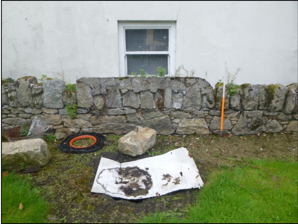
Plate 15 - Concrete mortar on granite boundary wall at location of underground structure (02.09.2019).
