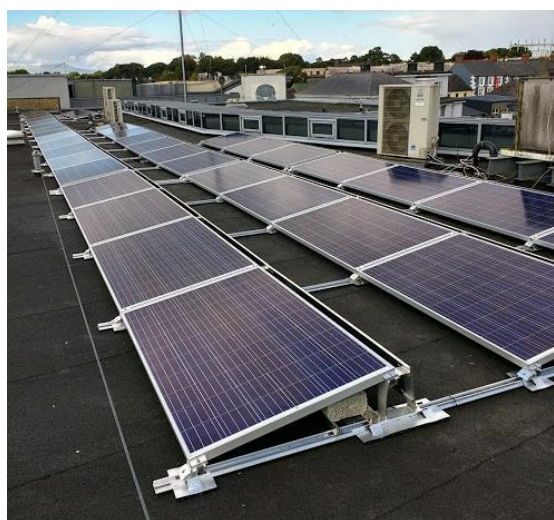
Figure 7.12: PV panels on roof of Tullow Area Office
