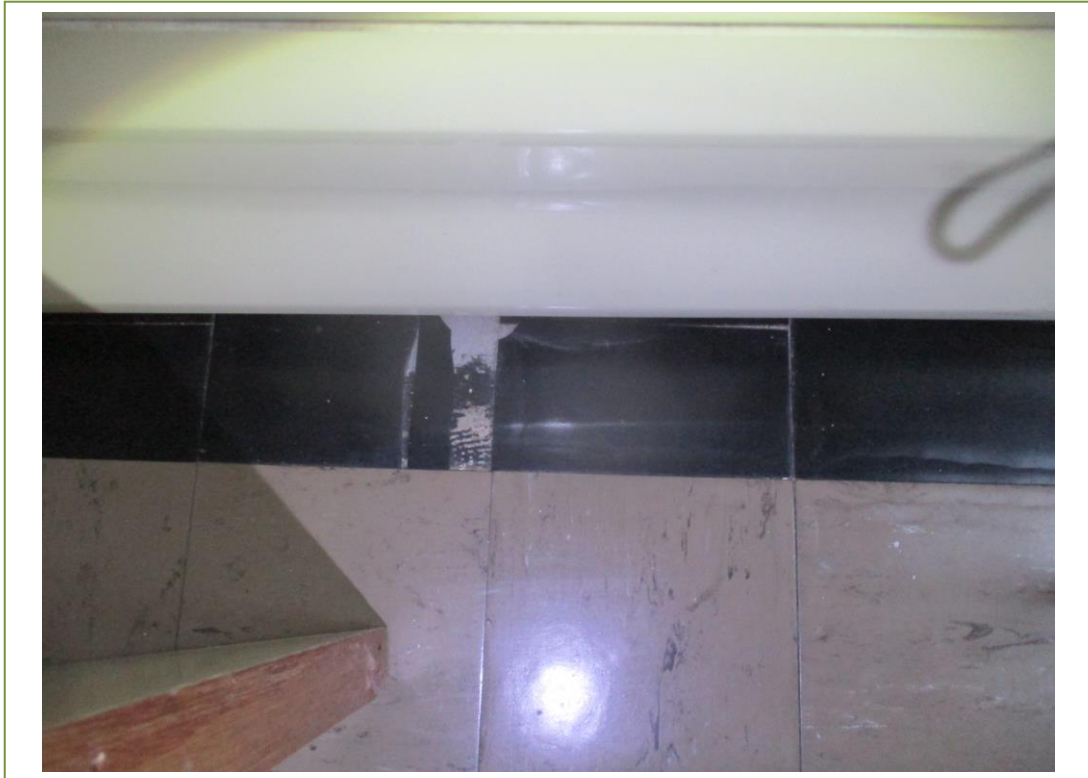
View of the asbestos containing floor tiles and bitumen adhesive in the toilet on the 1 st floor
