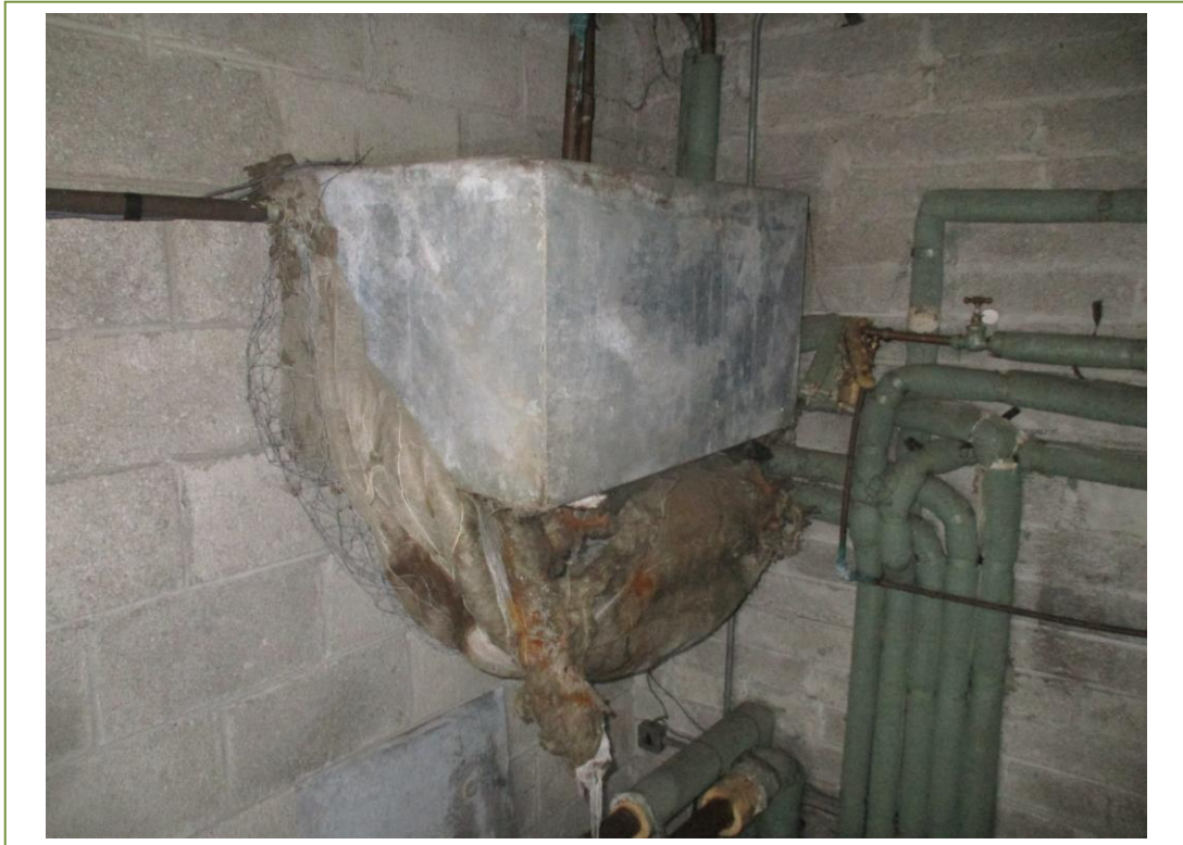
Steel water tank
