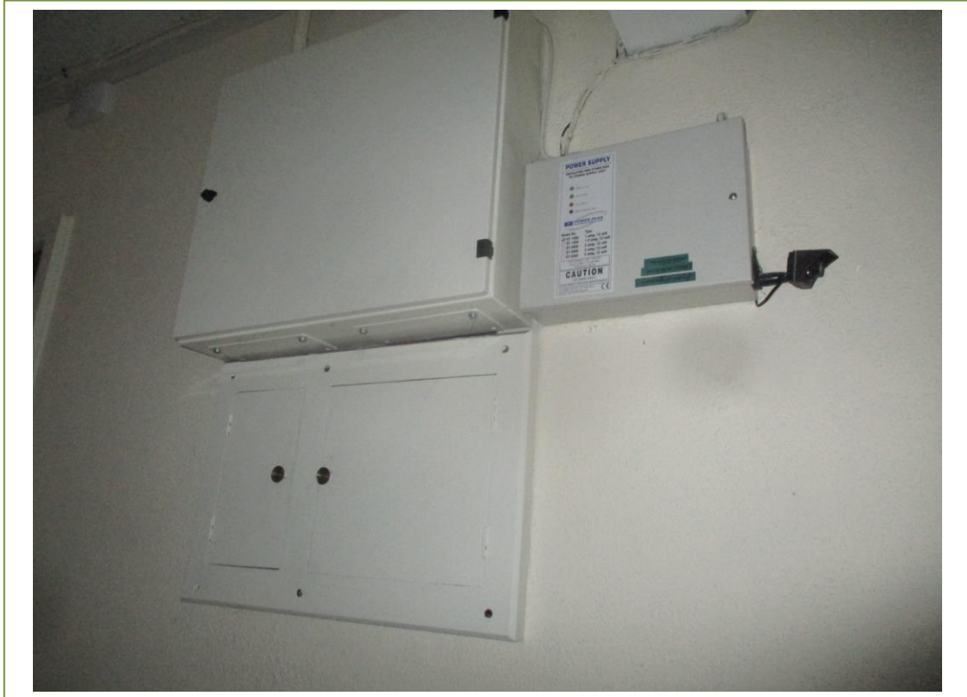
Modern Electrical unit
