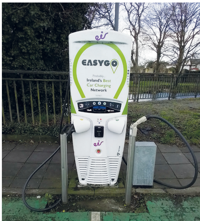
EV Charging Point at New Road, Tullow
