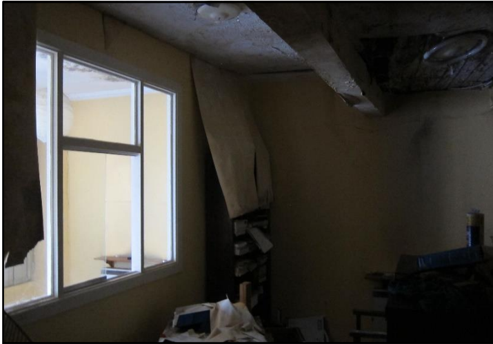
Plate 5: Derelict office (inside building)
